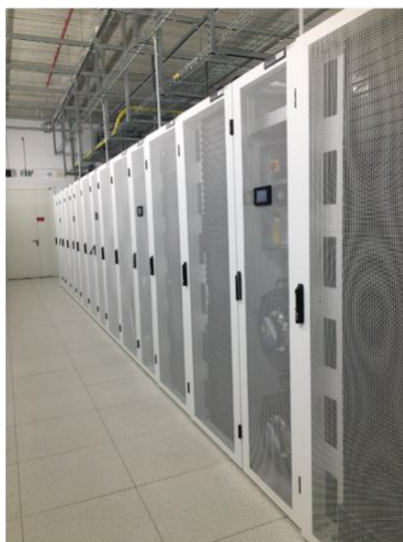
Explor Room @ Univ. Lorraine Datacenter
